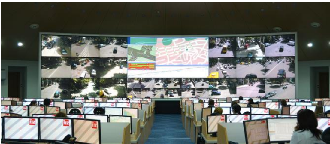
Picture 3. Tbilisi traffic lights control center.
