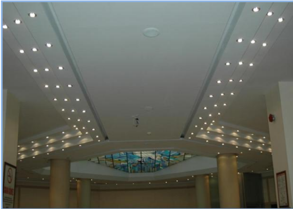
LED Fixtures- 5 watt
