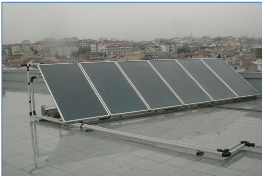
Picture 12- Solar Collector on the roof of Kadıköy Municipality
