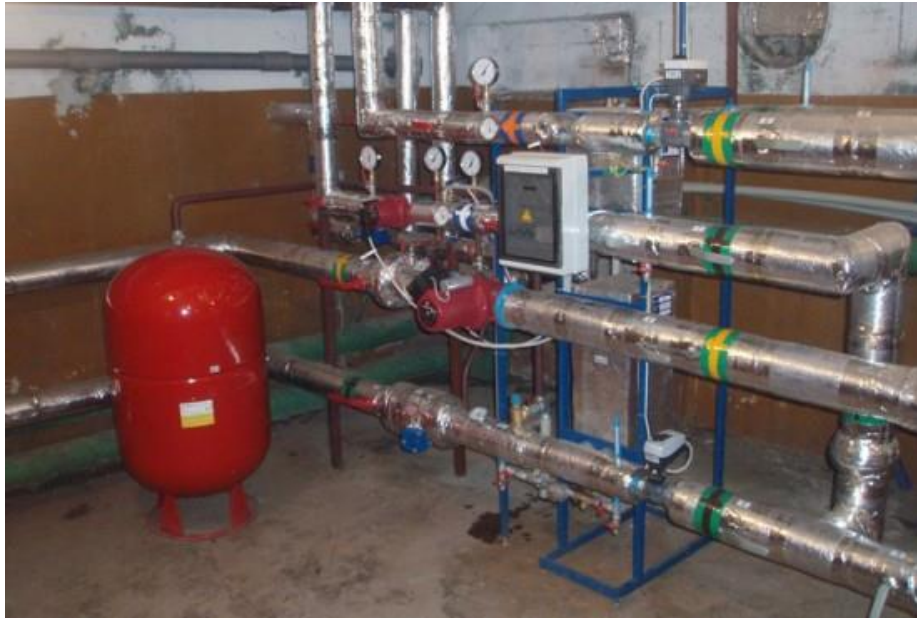
Image 9. Individual heating unit
