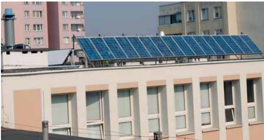
Solar panels on the building of the Schools Complex No. 113 with Bilingual Sections at Olgierda St. in Warsaw. Phot. from the archives of the Infrastructure Department
