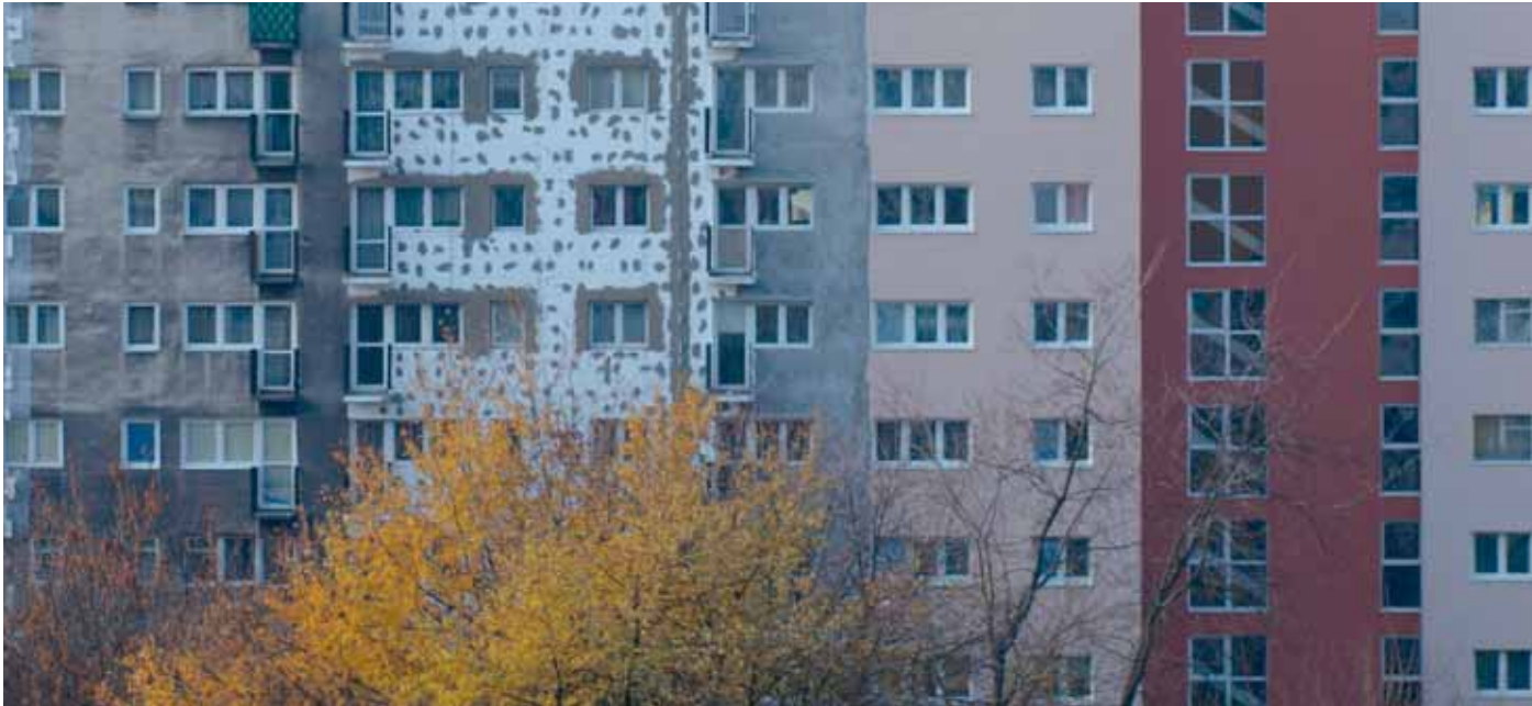
Works on thermal retrofit (insulation) of a residential building. Phot. from the archives of the Infrastructure Department.
