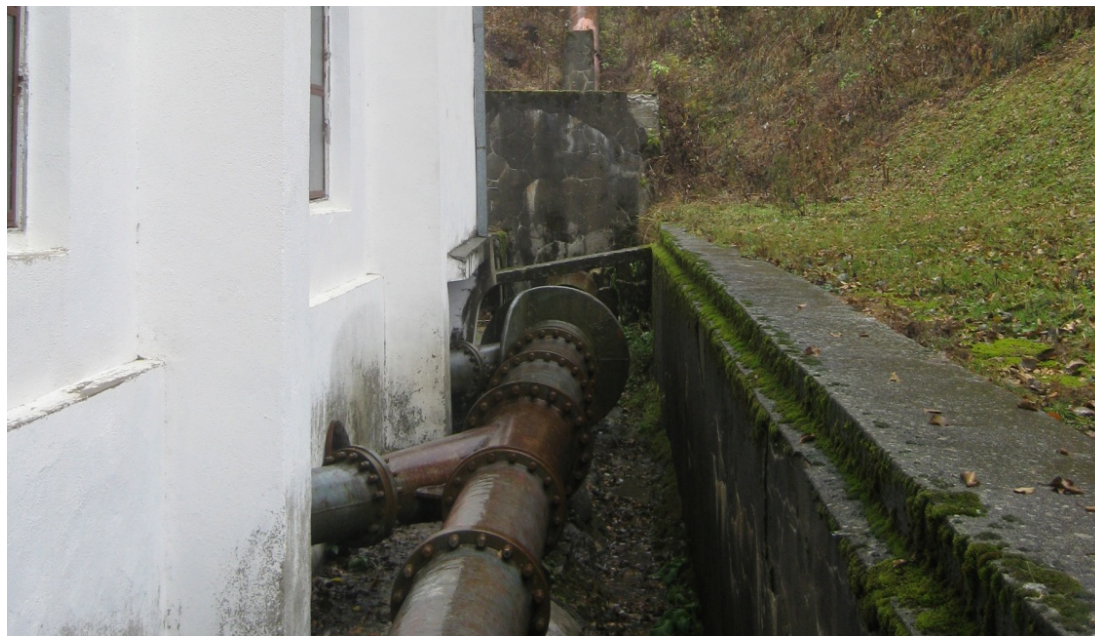
Figure 2.2: Detail of the Mušovića Rijeka Small Hydro Power Plant
