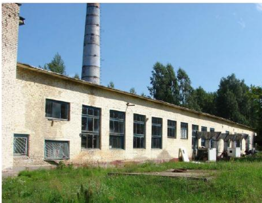
Figure 1. Boiler house “Borovukha-3”
